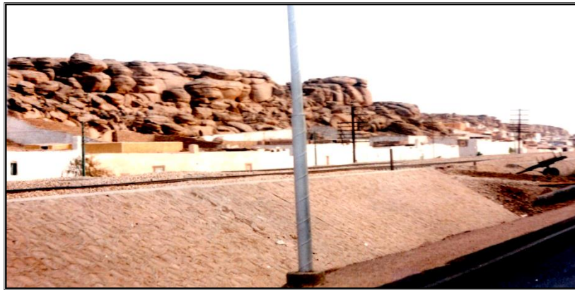
Photo 4. Vertical and horizontal cracks on the slope of the embankment (Village El Khatarah)
