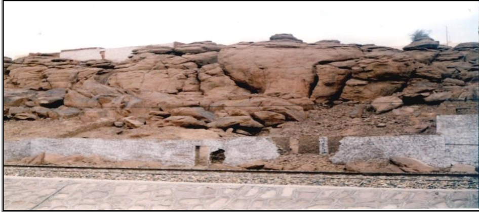
Photo 2. Thermoclasty in the eastern slope of the Eastern Slope (sandstone) north of Aswan.
